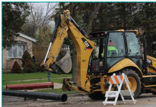
Utilities Division staff responded to eight water main breaks
