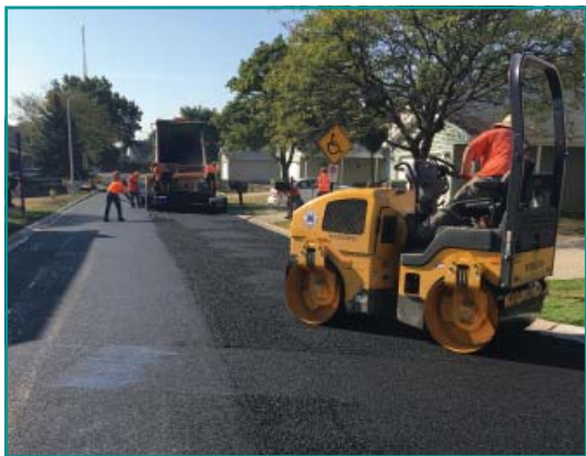
In-House Road Program Overlaying Wyatt Lane, Burr Oak Lane, Basswood Lane and Westchester Drive
