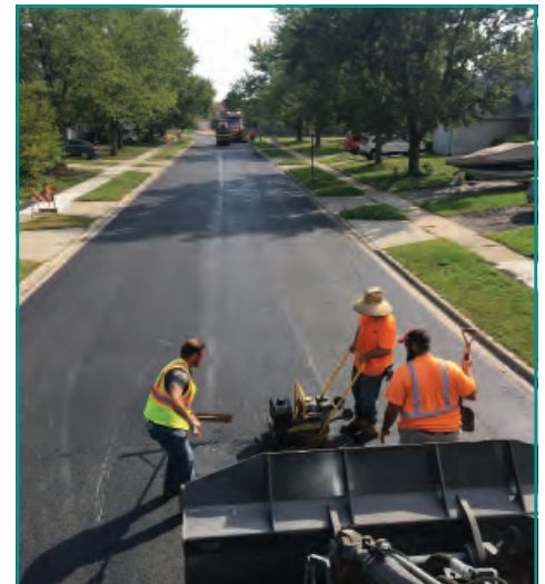
The in-house road program overlayed Fallbrook Dr., Floyd Brown Ln., Keating St., and Elizabeth Ave.
