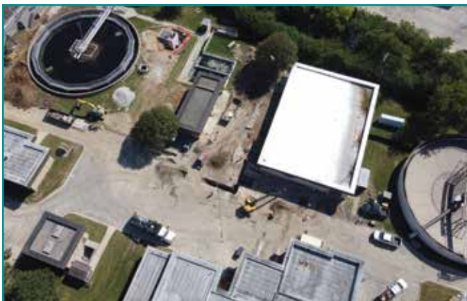
Capital improvements continued at the Wastewater Treatment Plant including rehabilitation to Digester #2
