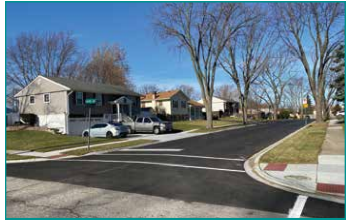
Eight streets were reconstructed as part of the Motor Fuel Tax Road Program
