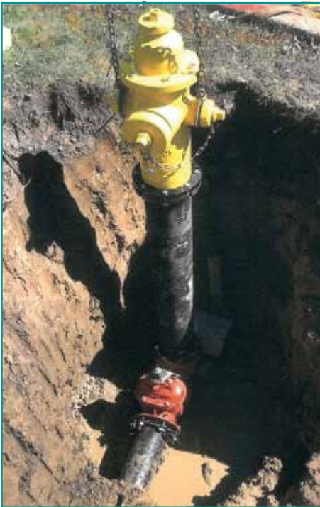
The Utilities Division replaced various fire hydrants to ensure they are in working order in the event of an emergency
